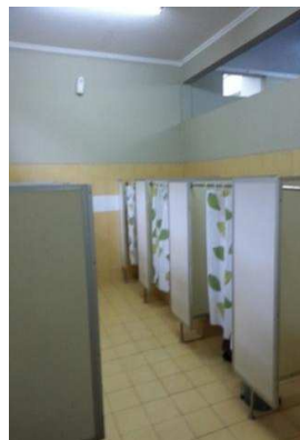
Gambar 2.132 Toilet Santa Laursenia
